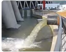
Power plant circulating water
