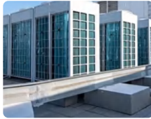
Central air conditioning
